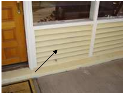
Louvers Front Exterior
