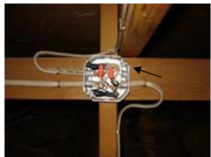
Open Junction Box
