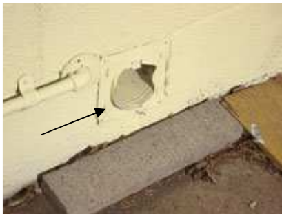
Dryer Vent Hood Missing
