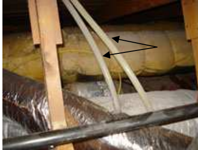
Attic Supply Piping Not Insulated
