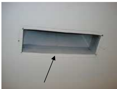
Ceiling Grills Missing Various Rooms
