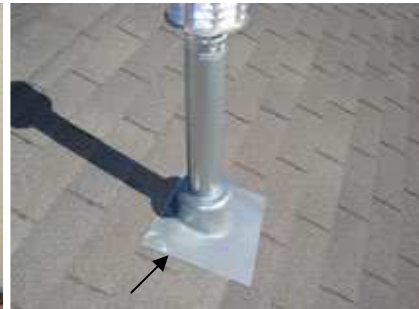
Water Heater Roof Flashing Exposed
