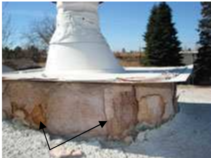
Deteriorated Flue Tile
