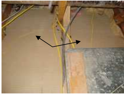
Missing Ceiling Insulation
