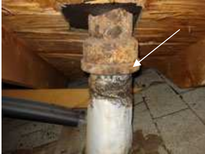
Plumbing Vent Loose Connection
