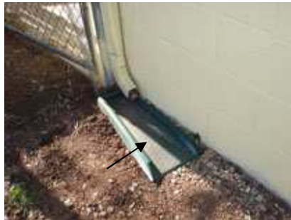
Downspout Discharge Next to House
